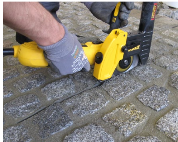
Cutting a movement joint into the road covering some days after the laying and jointing process.
