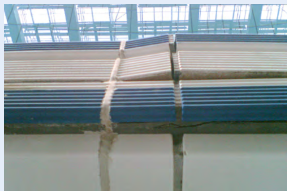
Damage due to insufficiently dimensioned movement joints in a swimming pool coping
