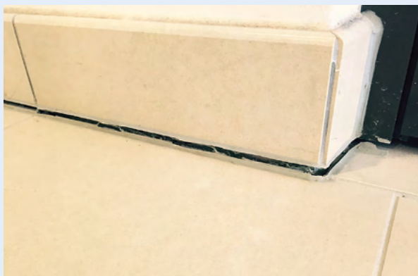
Overstretching of the sealant with cracking in the area of the skirting-wall connection
